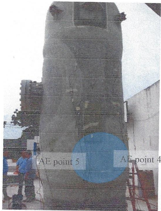
Figure 13. Position of AE indication revealed in Vessel 301 near AE point 5.
